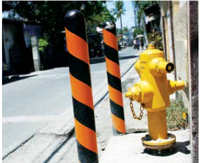
A typical fire hydrant installed by Laguna Water for the community along the coast of Laguna de Bay
