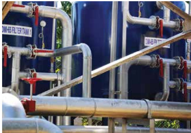
Laguna Water uses the DMI-65 Filtration System, a state-of-the-art device, to reduce manganese content in water.
