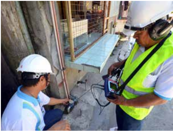
Leak detection teams regularly check service connections to prevent water loss resulting from pipe breakages.
